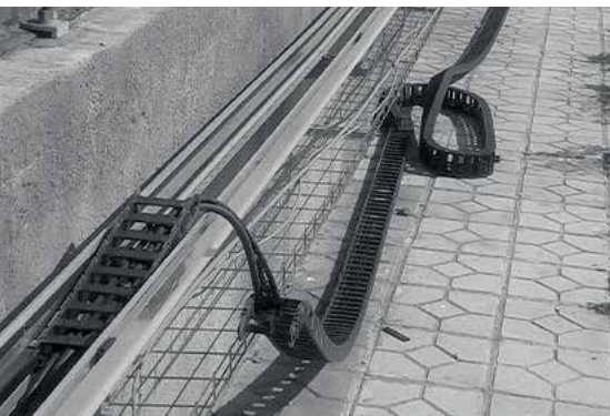
energy chain and cables destroyed by a blockage in the guide channel. Source: igus-
