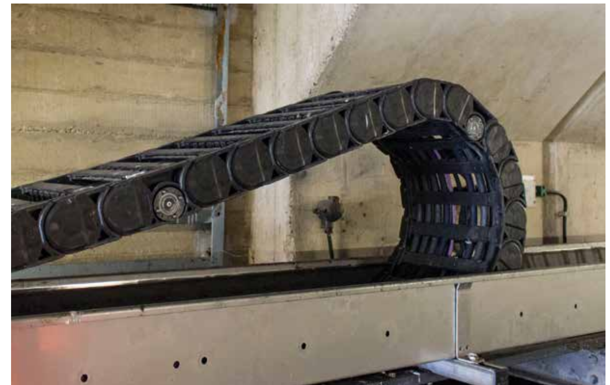
chainflex® Fiber Optic Cable in sea lock
