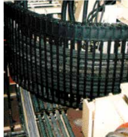
Hydraulics and electric cables are separated from one another in this example
