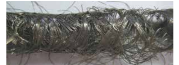
The detail inspection of the shield braid shows distinct damage on the shield wires.
