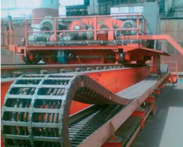
igus® rol e-chain® Series 5050R in a steel plant in India with highly corrosive atmosphere - Travel = 72 ft. (22 m), v = 3.28 \text{ ft/s} (1 m/s), a = 3.28 \text{ ft/s}^2 (1 m/s 2 )
