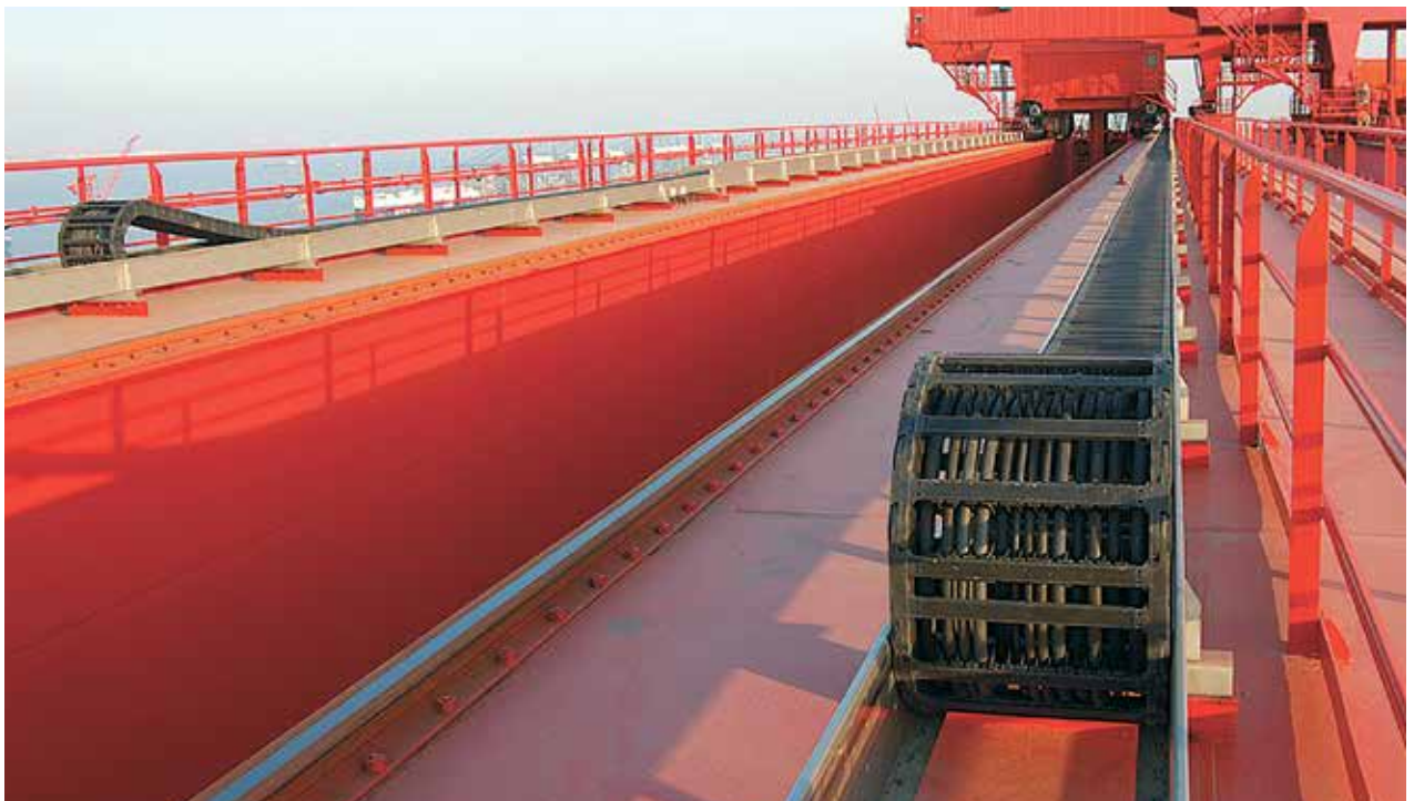
Shipyard-Crane: 590.5 ft. (180 m) travel, 20.16 lbs/ft (30 kg/m) fill weight: No problems since installation in 2001 with igus® rol e-chain®
