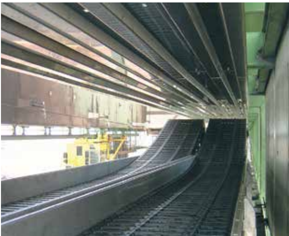
Assembled system in a ship unloading crane with igus® 5050RHD - Travel 248 ft. (106 m), Speed 13.12 ft/s (4 m/s), Fill weight 16.8 lbs/ft (25 kg/m)
