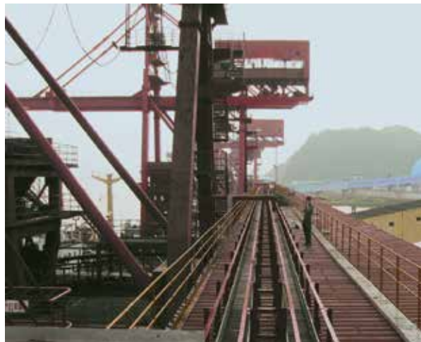
Series 4040R on a coal unloading system - Travel 623 ft. (190 m), Speed 1.6 ft/s (0.5 m/s), Fill weight 5.41 lbs/ft (8.05 kg/m)
