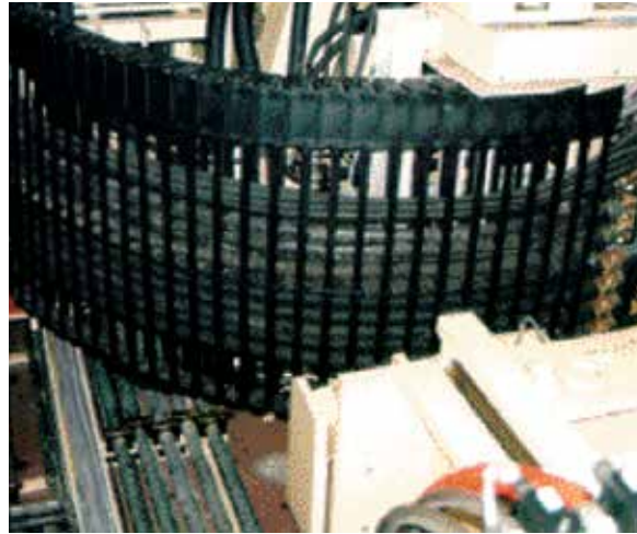
Hydraulics and electric cables are separated from one another in this example
