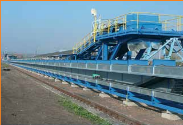
The world's longest e-chain® travels 2017.8 ft. (615 m) with igus® rol e-chains® and chainflex® cables in a power plant
