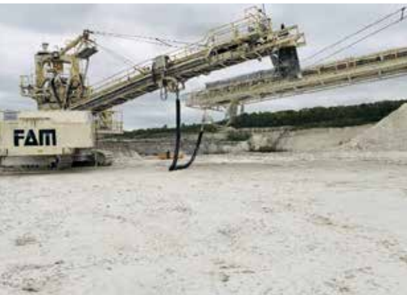
Picture 7 In this application, the e-loop® is sometimes hanging and sometimes on the ground, depending on the excavator boom condition. Source: Holcim/igus® GmbH
