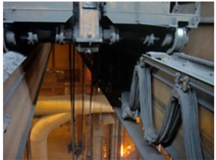
Energy supply via open hanging festoons on a two-girder crane.
