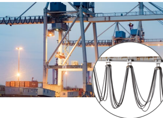
In cable trolley systems (festoons), the cables "hang" from the cranes, unprotected from wind and weather. Source: Fotolia and igus® GmbH
