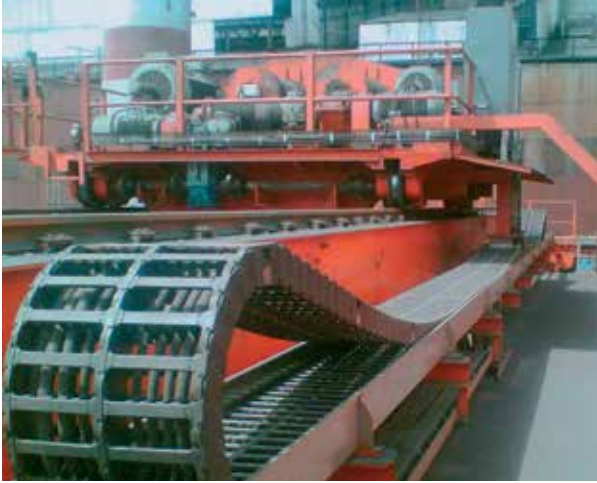
igus® rol e-chain® Series 5050R in a steel plant in India with highly corrosive atmosphere - Travel = 72 ft. (22 m), v = 3.28 \text{ ft/s} (1 m/s), a = 3.28 \text{ ft/s}^2 (1 m/s 2 )
