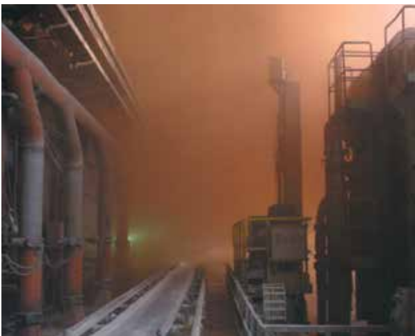
Series 4040R in steel works environment - Travel 34.5 ft. (10.5 m), Speed 197 ft/min (60 m/min), Fill weight 4.09 lbs/ft (6.084 kg/m)
