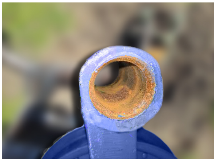
Result of a housing without corrosion protection
