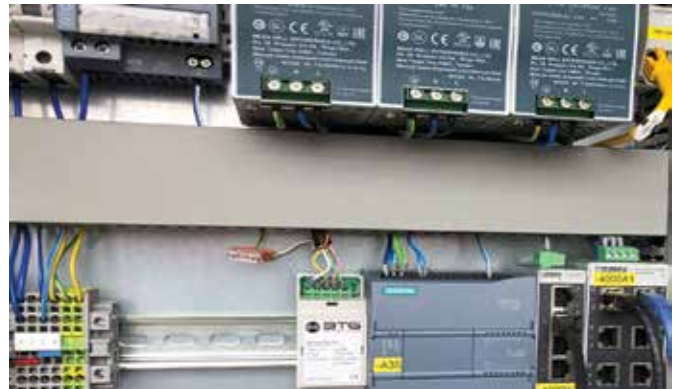
Switch cabinet with smart plastics modules
